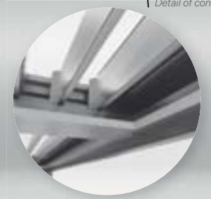
Detalle unión Vigas Centrales con Viga Plus Detail of connection between Central Beams and Plus Beam
